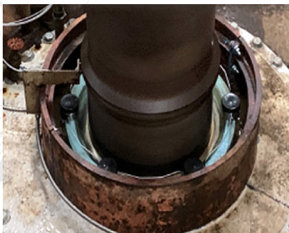
AMPS Technology in operation since April 2021.
